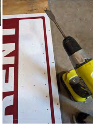
2. Lay flat onto scrap wood and use a spade bit to drill holes
